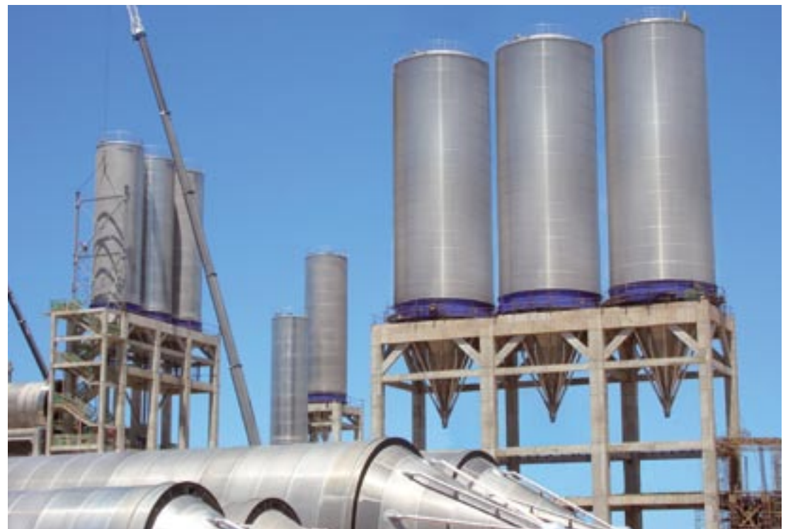
Plant with aluminium Multi- Channel Blenders with a capacity of 2850 m 3
